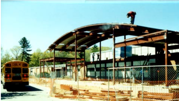
View of the new, steel framed barrel roof at the addition to the front of the school under construction.
