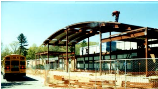
View of the new, steel framed barrel roof at the addition to the front of the school under construction.
